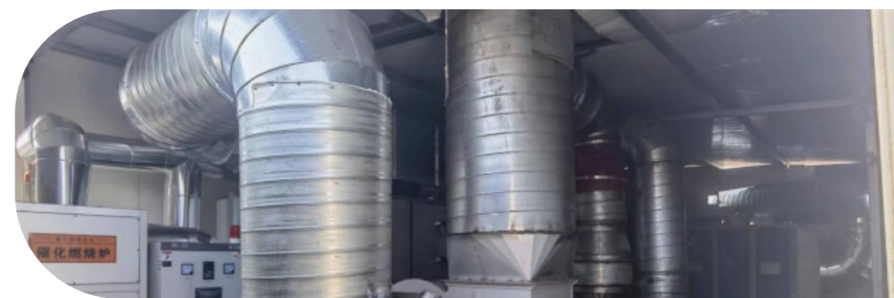
Waste disposal equipment
