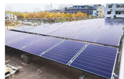
In November 2020, he served as the No. 12 Middle School in Xiangyang, Hubei Donated 60kW rooftop photovoltaic, the project started It will be connected to the grid in February 2021, with an annual power generation capacity of 60,000 kWh.
