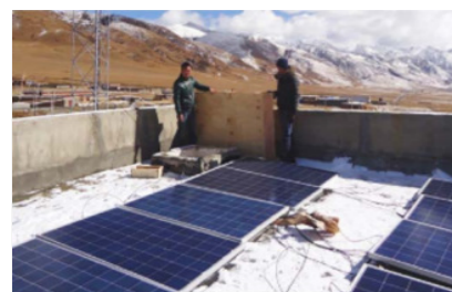
In October 2013, Seraphim provided services to Litang, Sichuan County Heni Township Primary School and Pajiang County, Zhongba County, Tibet Township primary school donated 5KW solar photovoltaic power station.
